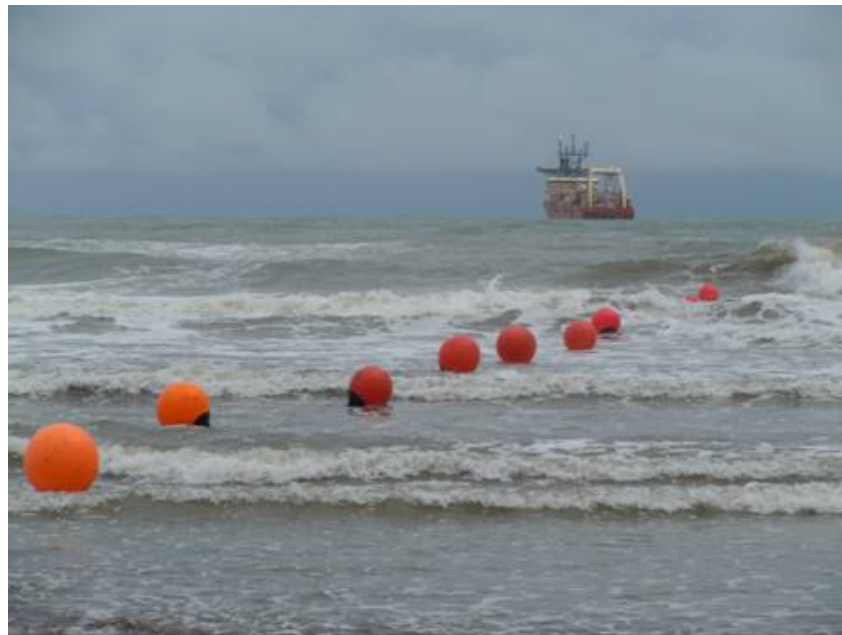
Shown in photo is the cable ship, C/S Fu Hai, laying out the ASE cable which was floated to the shore using the orange buoys.
